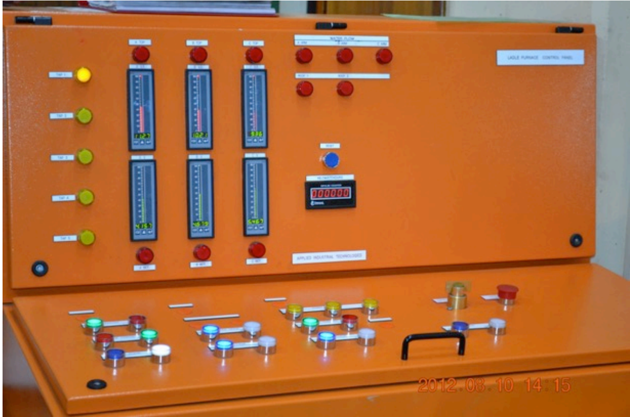
Example of a control cabinet
